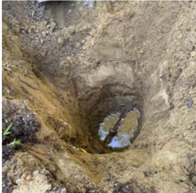
Example image of potholing to reveal a curb stop and identify water service material.
